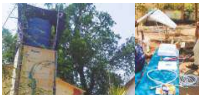
Mobile Booster Installation Vangani Ashram School, Maharashtra
