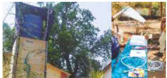
Mobile Booster Installation Vangani Ashram School, Maharashtra
